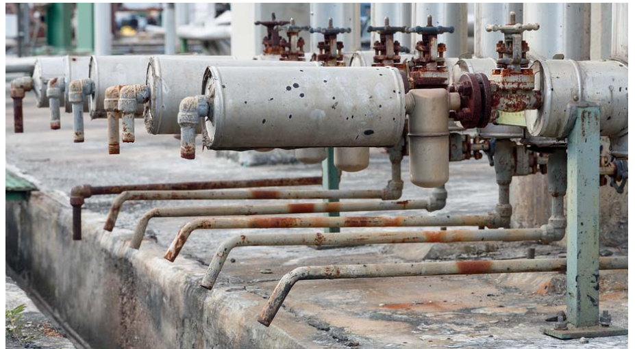
Old steam traps in an industrial plant – a clear indication that although steam is a fluid of very significant importance in our industrial plants, managers do not often give it the attention it deserves, particularly when the apparatus that uses it may be regarded in the factory as 'critical' equipment.
